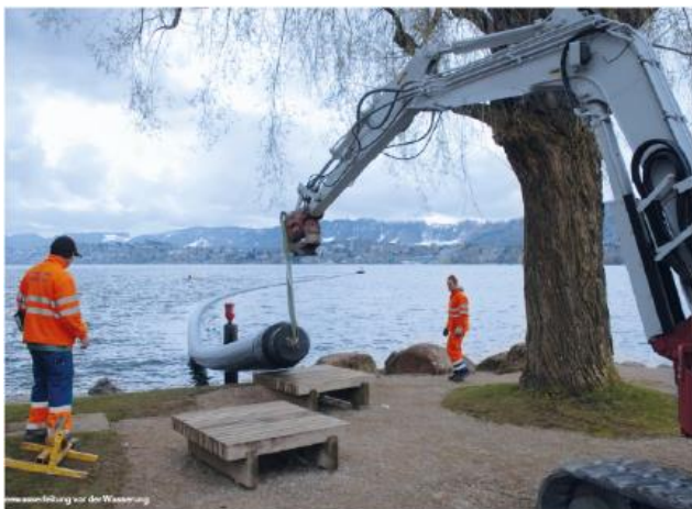
picture: construction of lake water pipeline that transports the water to the energy network power station
